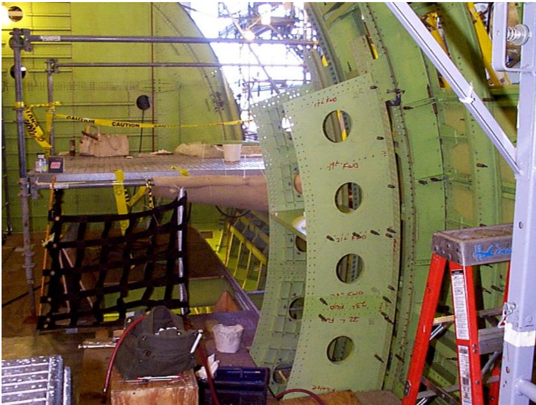
Figure 7.7-33. In Waco, the bulkhead installation begins. The view from the cabin looking aft into the cavity area – July 2002.
