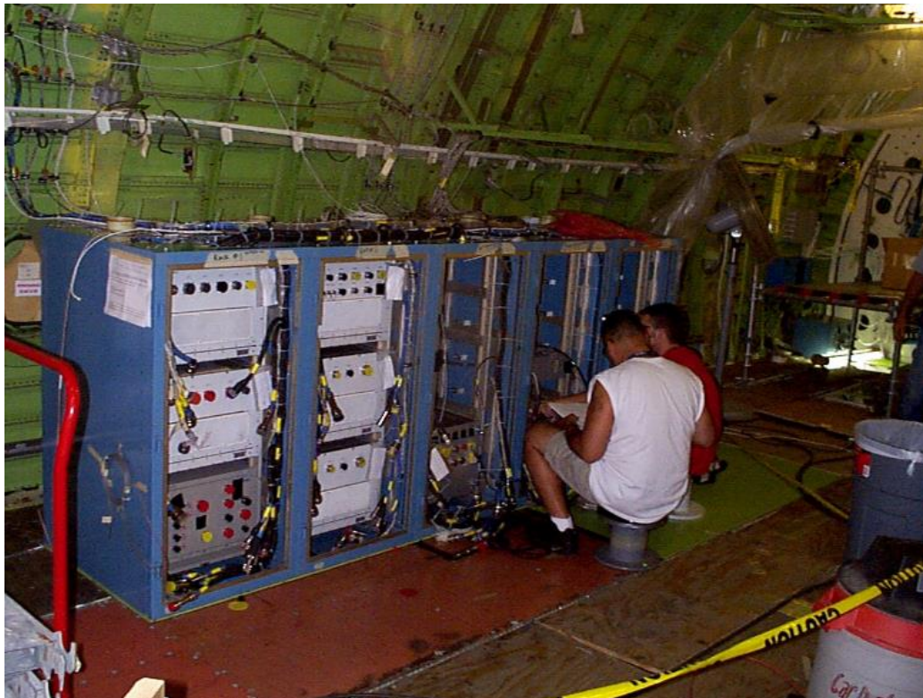
Figure 7.8-30. The aft racks that are part of the telescope being installed and hooked up – August 2003.
