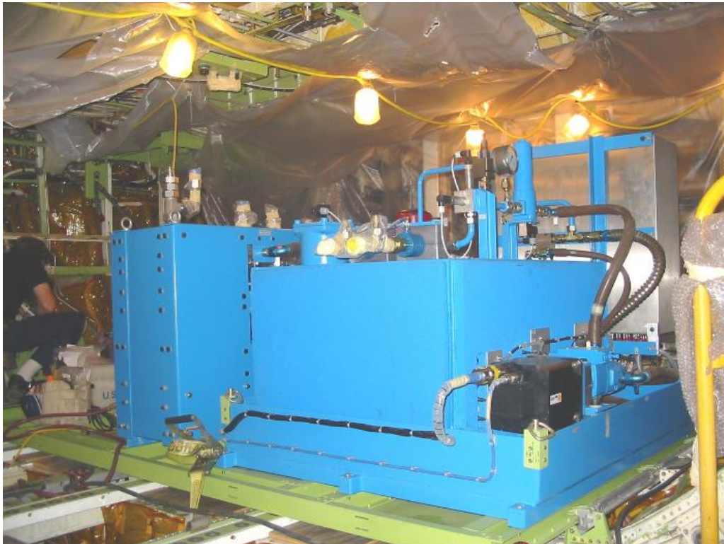
Figure 7.8-28. Another TA support system (the hydraulic system for the RIS) on a pallet installed in the forward part of the forward lower cargo bay (under the main floor) – July 31, 2003.
