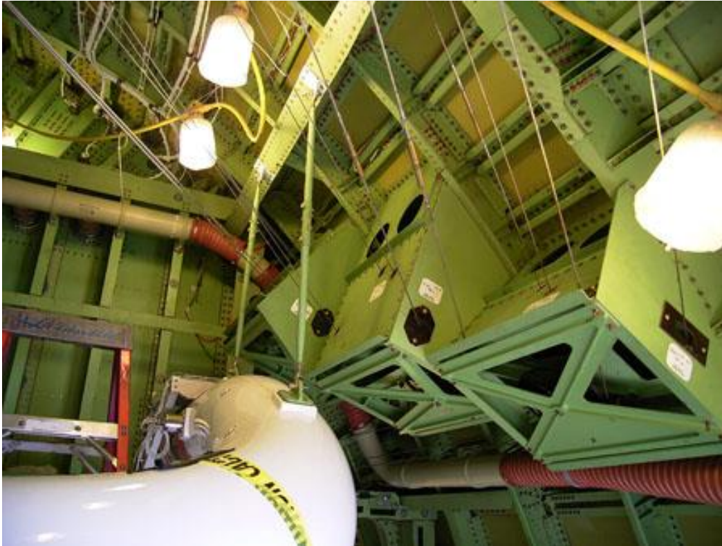
Figure 7.11-3. Control cables for the empennage: this view is from the fuselage area aft of the telescope cavity looking forward where you can see the control cables that are re-routed from near the top center of the fuselage to lower down on the right side – January 2006.
