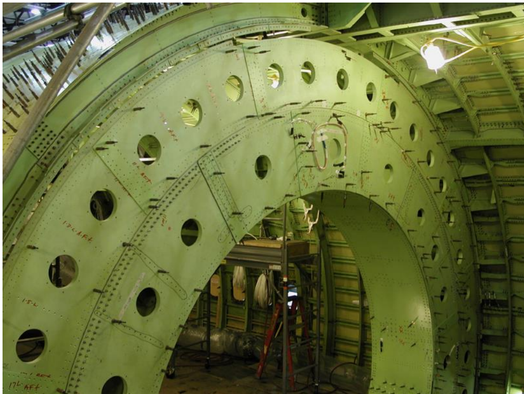
Figure 7.7-46. Status of the pressure bulkhead installation where the telescope will be mounted, looking forward from the cavity area into forward fuselage – October 2002.
