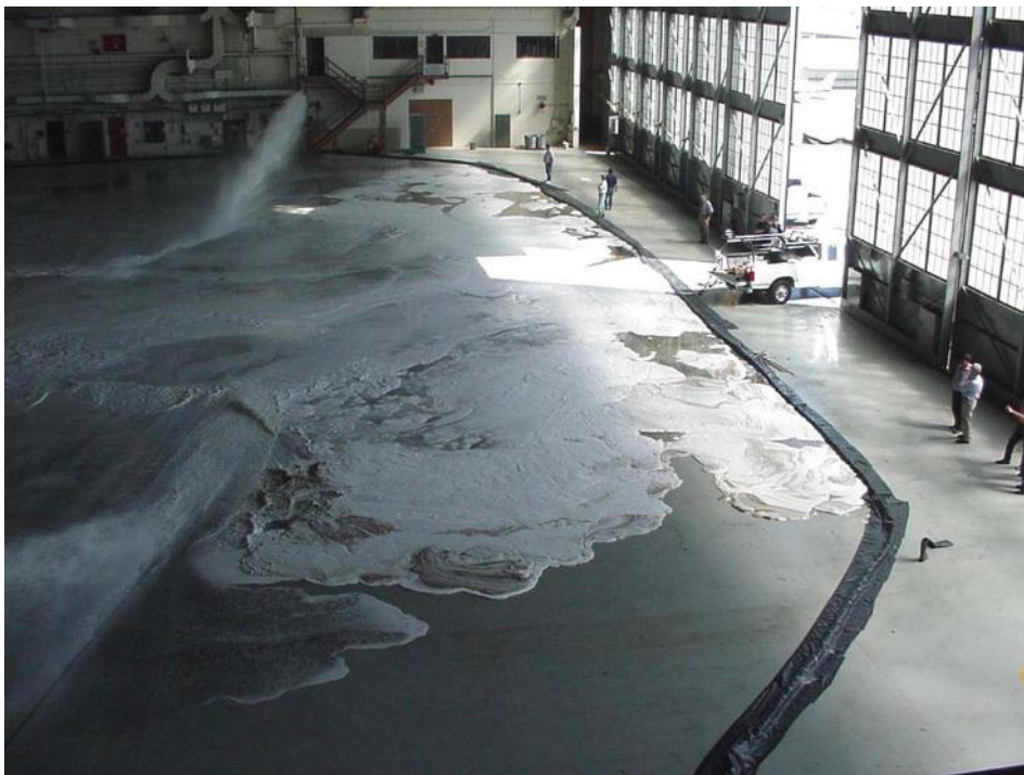
Figure 7.6-18. The inside of N211 during the verification test of the newly updated fire suppression system – June 2001.
