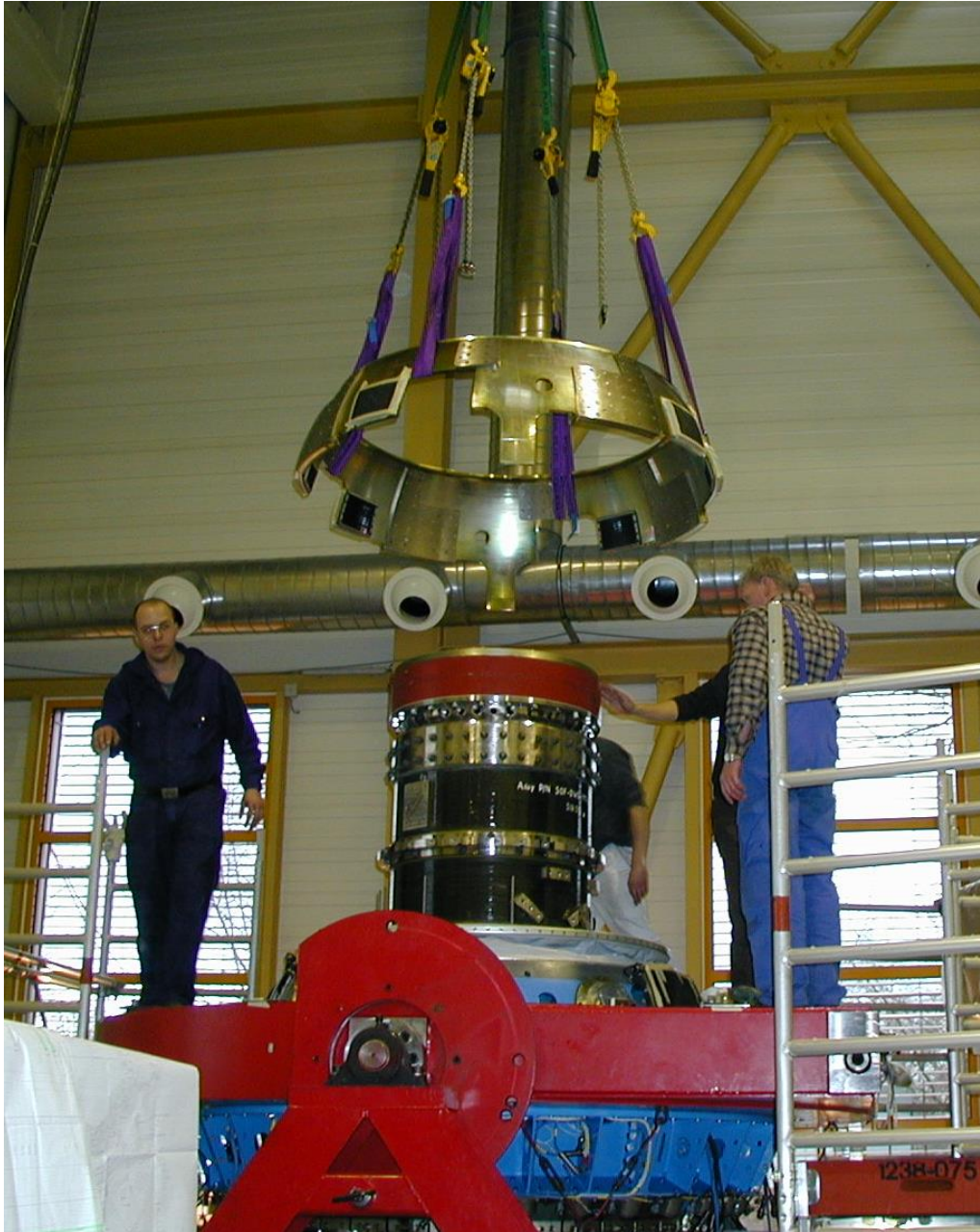
Figure 7.6-42. Another layer of the SUA being installed on the cabin side – December 6, 2001.
