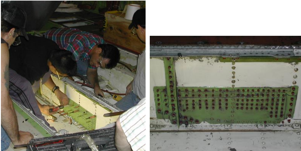
Figure 7.9-5. Photo on the left is the crew working on this repair; on the right is the finished repair (April 24, 2004) just a few hours before the proof pressure test.
